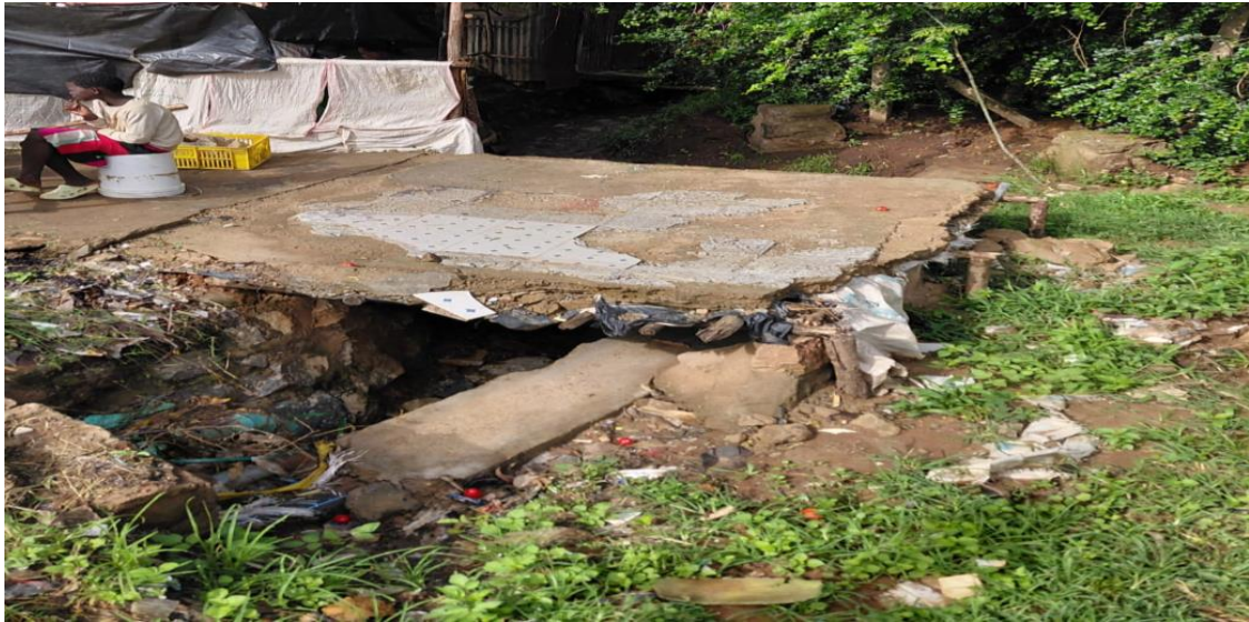
Plate 7: Liquid effluent from the road adjacent to the corridor being discharged on road reserve
