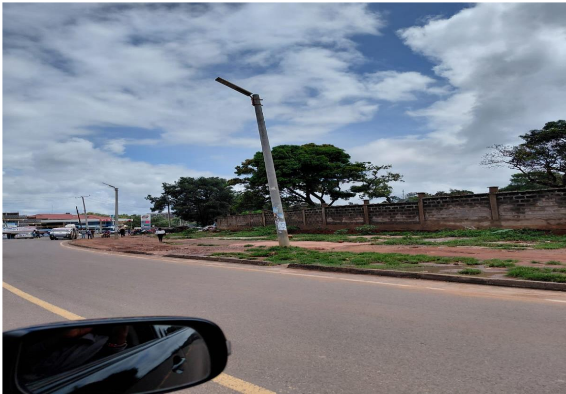
Plate 14: Street lighting along the corridor proposed for improvement
